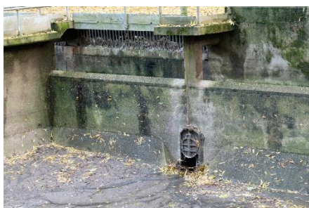
Ewell Storm Tanks
