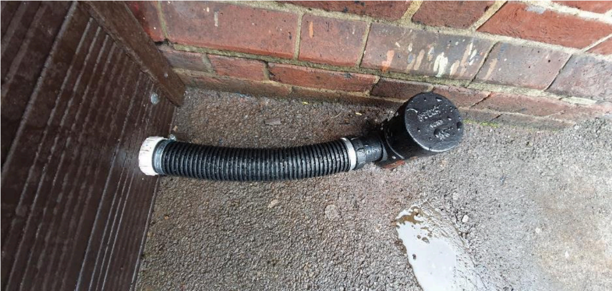
Figure 20: Planter outflow connected to the downpipe by a mechanical soil boss connector.
