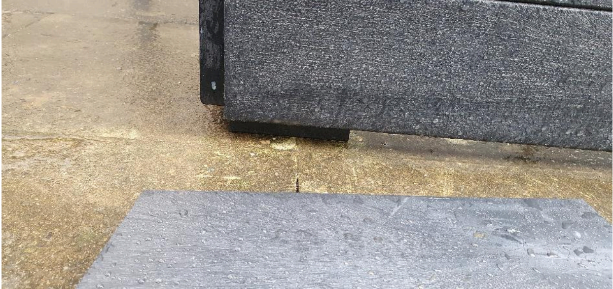
Figure 32: Note the gaps left when fixing the supporting blocks so a covering strip can be installed.
