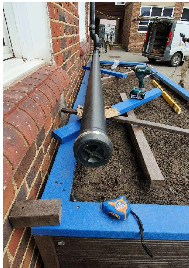
Figure 13: Temporarily connected distribution pipe and held levelled before marking the final position of the brackets.
