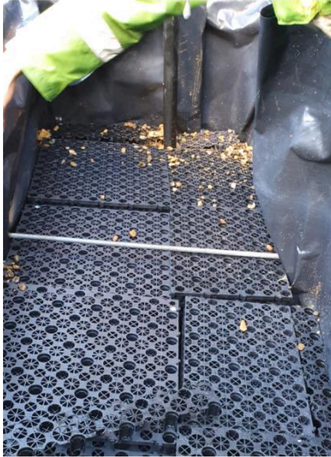
Figure 23: Note the offcuts used to cover the gap on the right hand side, and the gravel filling the voids close to the draining pipe.
