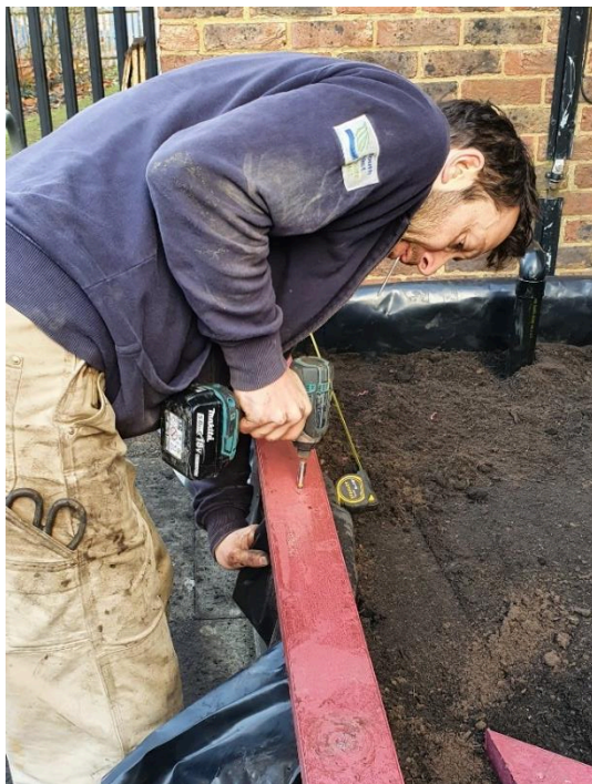
Figure 47: Rim installation, note how the membrane is being pulled while the rim is being fixed into place.
