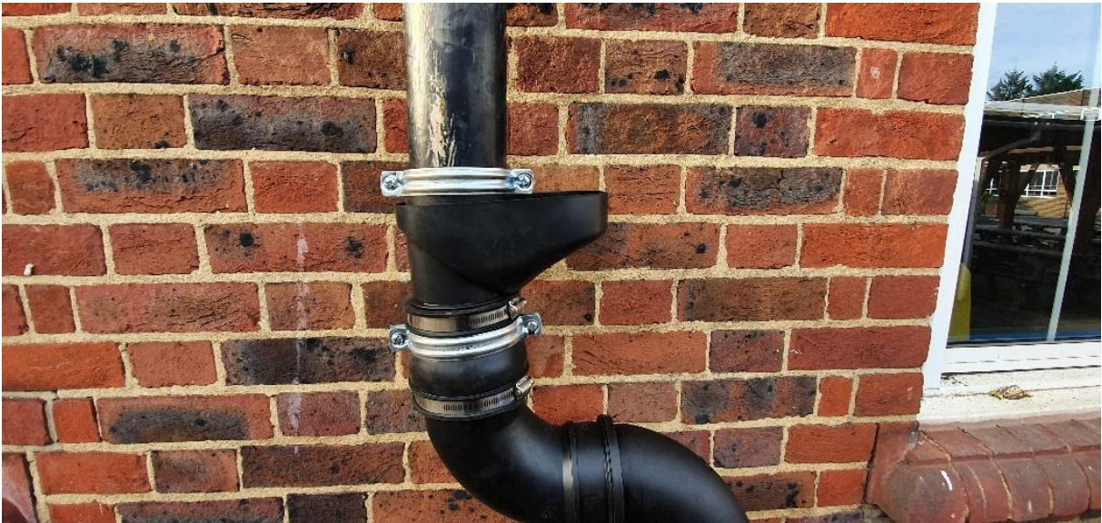
Figure 15: Leaf filter being installed, it will make maintenance easier and reduce the risk of blockages in the raining pipe.
