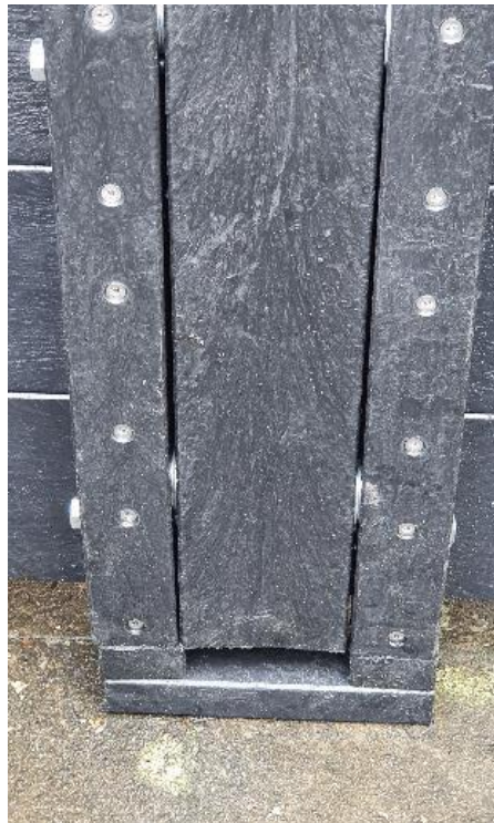
Figure 31: Fixed chocks in the centre joints.
