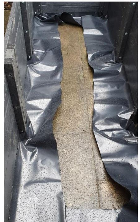
Figure 34: Pond liner skirt installed to keep the protective layer of sand inside the planter.
