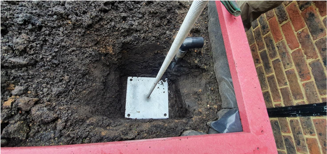
Figure 16: Position of the base of the arch attached to a threaded bar.
