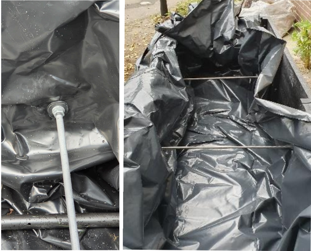
Figure 39: Installed cross bar with added sealant for creating a waterproof seal, and completed installation of cross bars in a planter.
