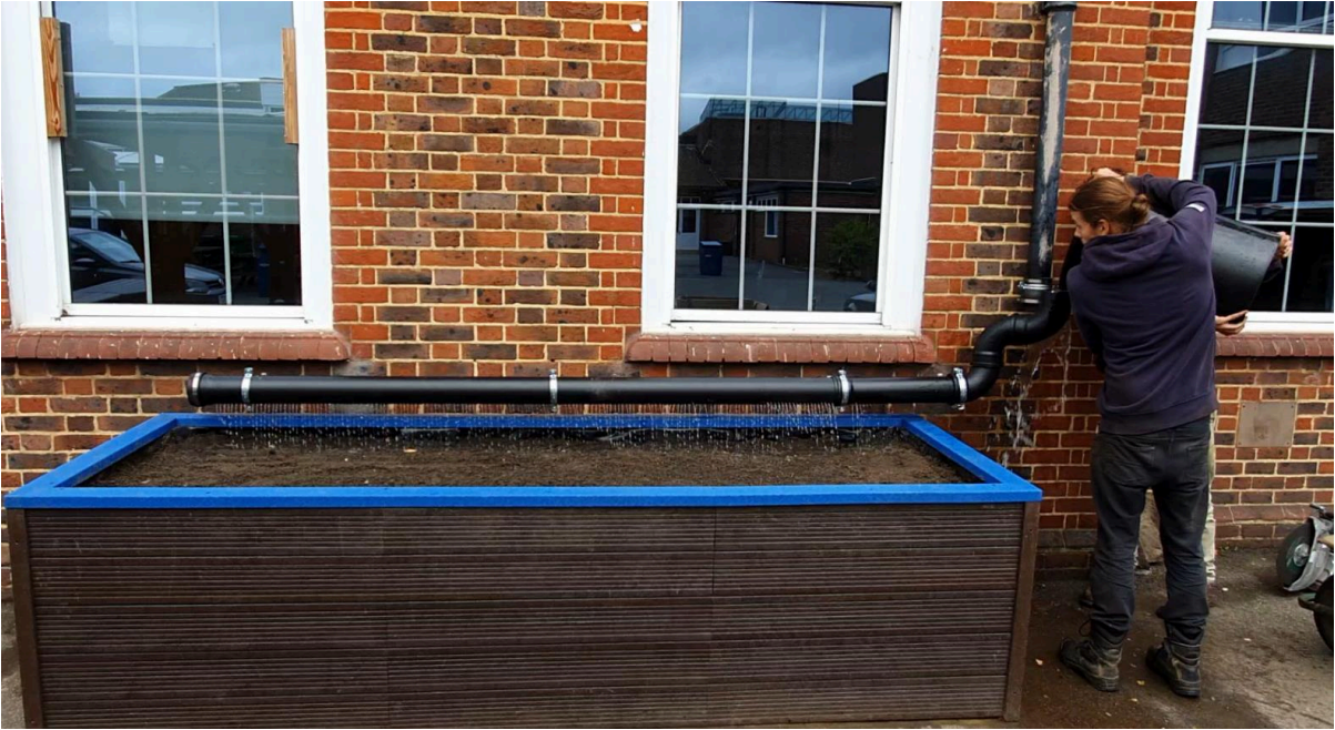
Figure 14: Checking the correct functioning of the distribution pipe. Note the symmetry between the brackets, and the brackets holding the cast iron down pipe and the elbow fittings.
