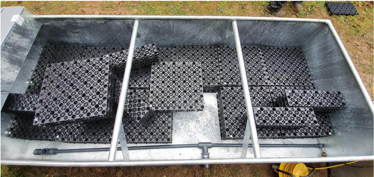
Figure 3: Installed configuration of the metal planter. Note the position of the outflow and how it affected the pipe connections and fittings.
