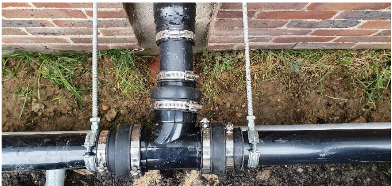
Figure 7: Different configuration of the distribution pipe due to the position of the downpipe in relation with the planter.
