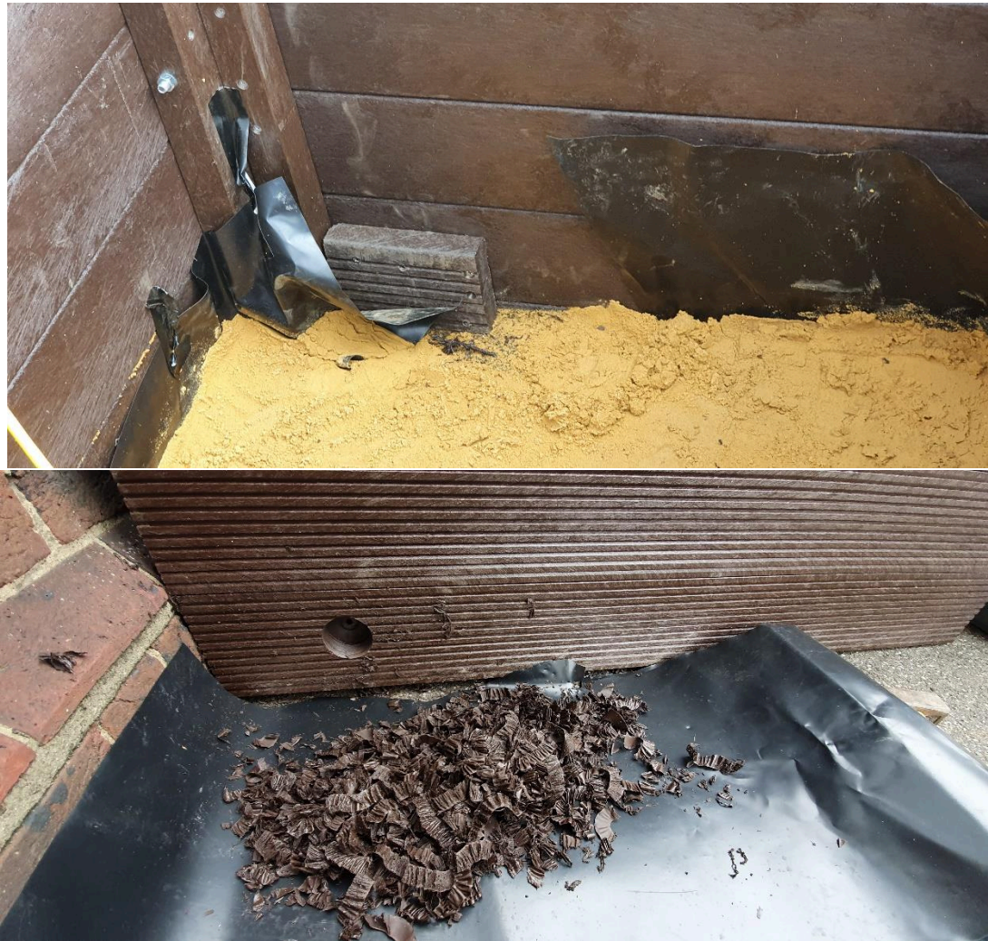
Figure 41: Temporarily fixed timber piece to allow the use of the adjustable auger bit. Note how the small pieces of plastic are collected and disposed of.
