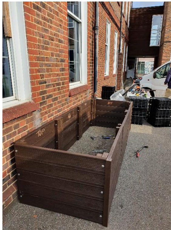
Figure 26: Chosen position of the planter after considering the position of the downpipe, the ground levels, and the visual symmetry in relation with the architecture.
