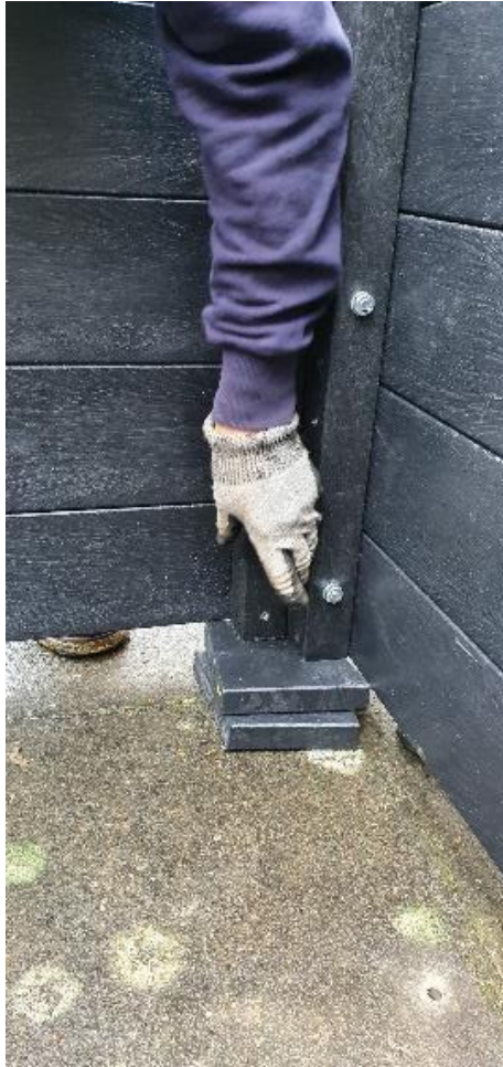
Figure 28: The planter is being temporarily supported so the gap can be measured and a chock can be cut and fixed.
