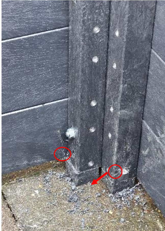
Figure 29: Fixing the chocks to the planter structure. Note the angle in which the screws were inserted.
