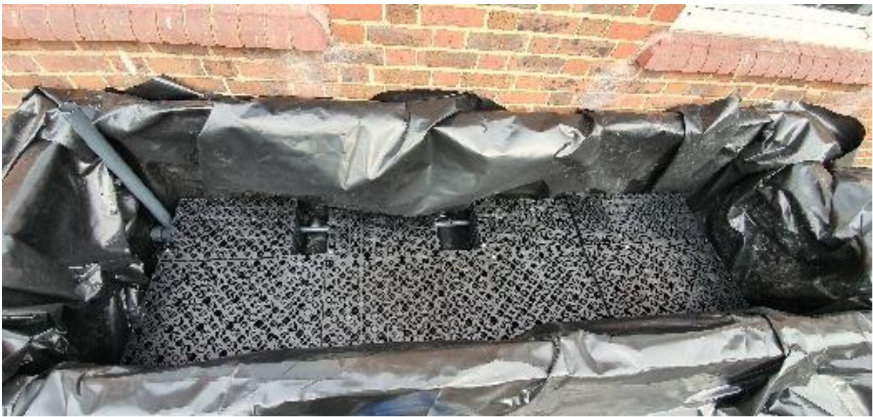
Figure 50: Installing the geocellular crates in the benched planters, note the different cutting and positioning of the crates.
