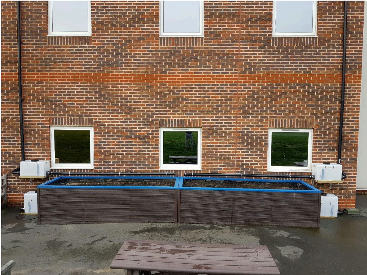
Figure 3. Monitoring set-up following installation. The figure shows the monitoring boxes upstream and downstream of both plants; one with a gravel sub-base, one with a geo-cellular crate sub-base
