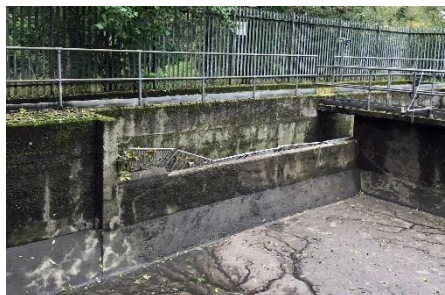
Ewell Storm Tanks (Photo thanks to Robb)
