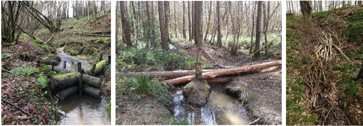
Figure 50. (Left and centre) LWSs installed in Pembury Walks and on the more incised stream south of the A228. Far right: Gully stuffing in the headwaters at Pembury Walks.
