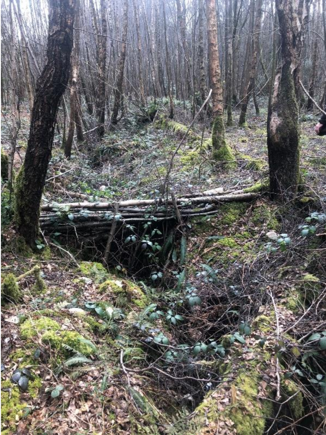
Figure 22. A LWS installed on the water course in Bedgebury Forest. The photo shows that the stream was quite incised prior to installation, especially relative to the width of the stream.
