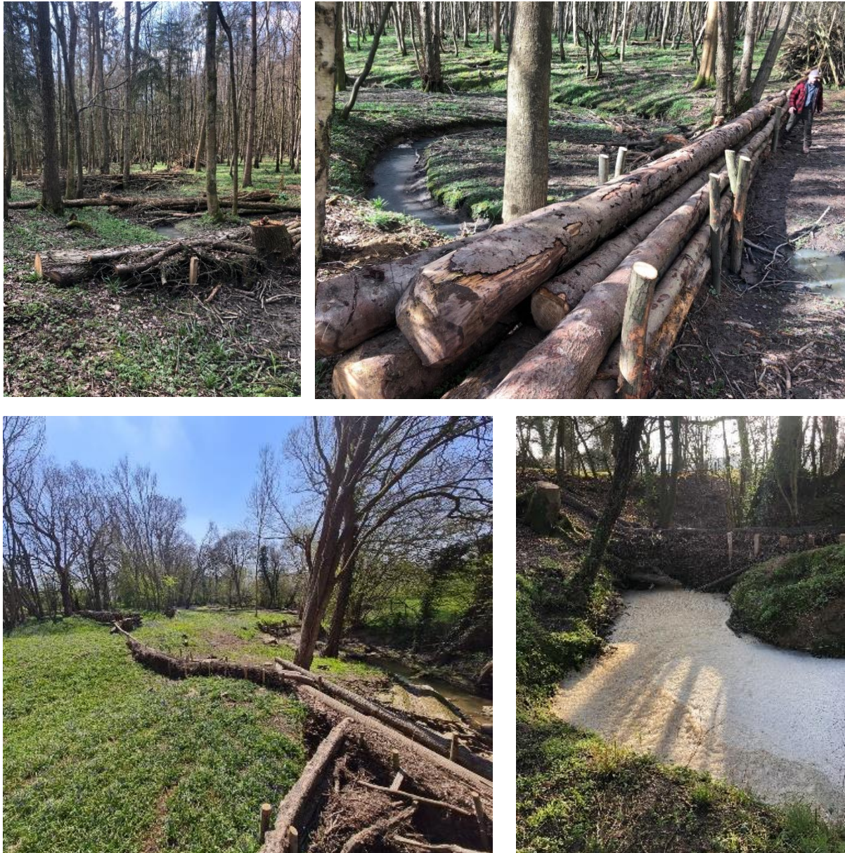
Figure 71. Series of large LWSs installed on eastern tributary in Birch Wood (top). LWSs constructed at Stonehall Farm (bottom), including one braced against the historic dam on the site (bottom right).
