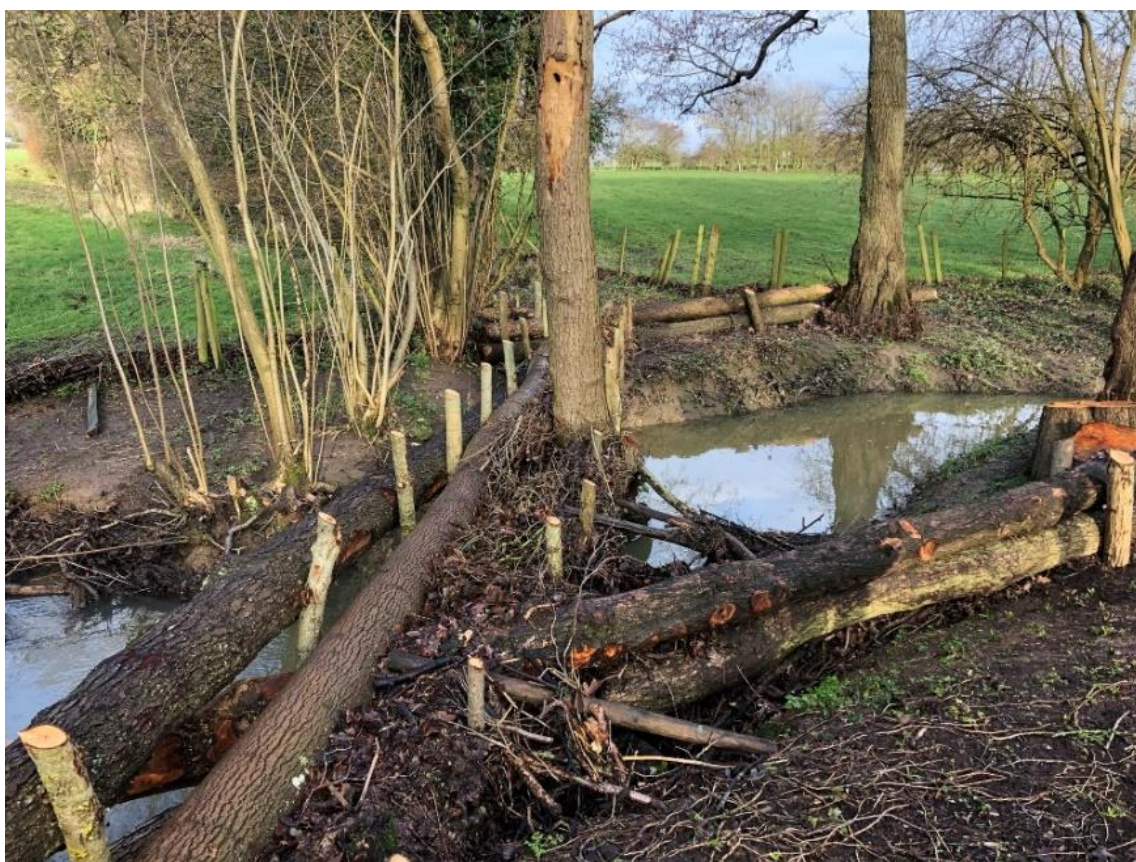
Figure 78. LWSs at Stonehall Farm, enhanced with faggot bundles, became even more effective at trapping silt and debris
