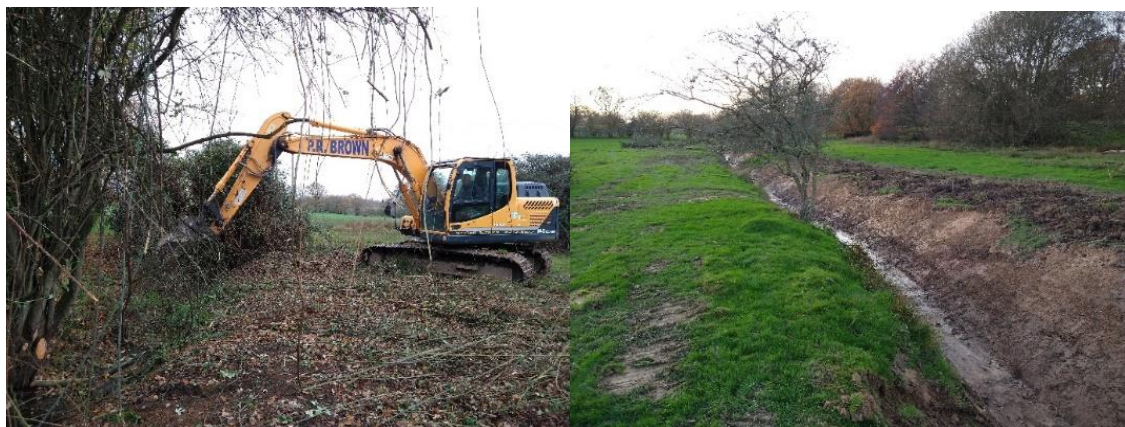
Figure 53. Left: Excavator removing soil and silt from the southern ditch to restore its capacity. Right: Fully restored ditch.
