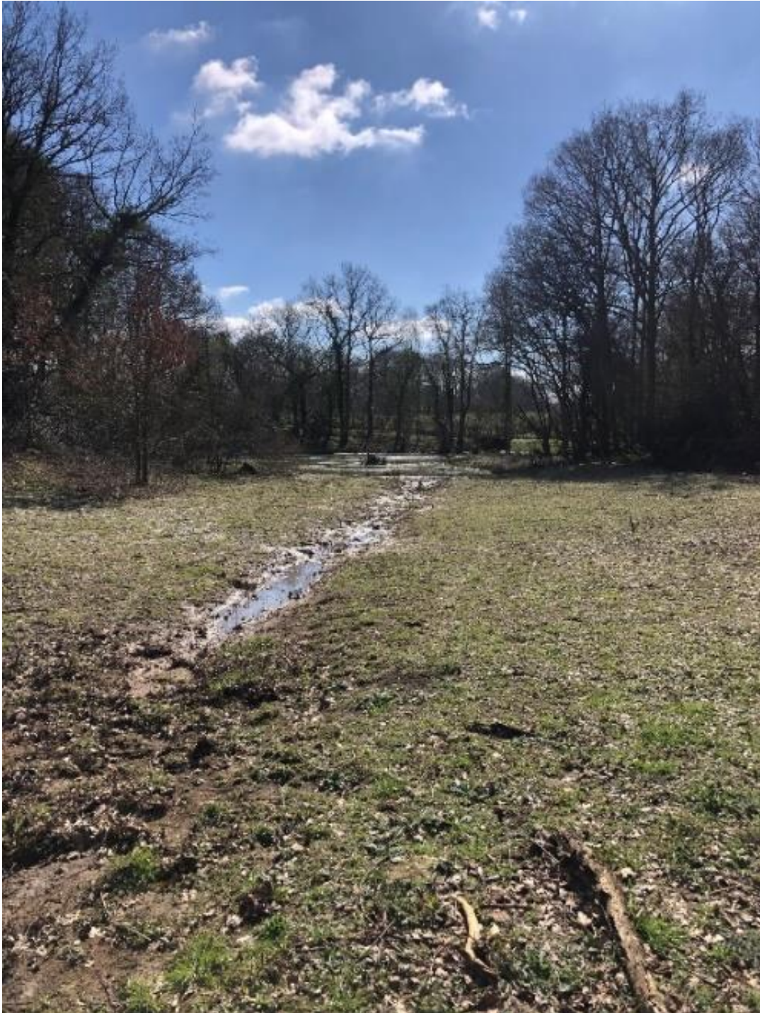
Figure 84. The spillway to Kingsnood pond has accumulated noticeable levels of silt in the year following its installation.
