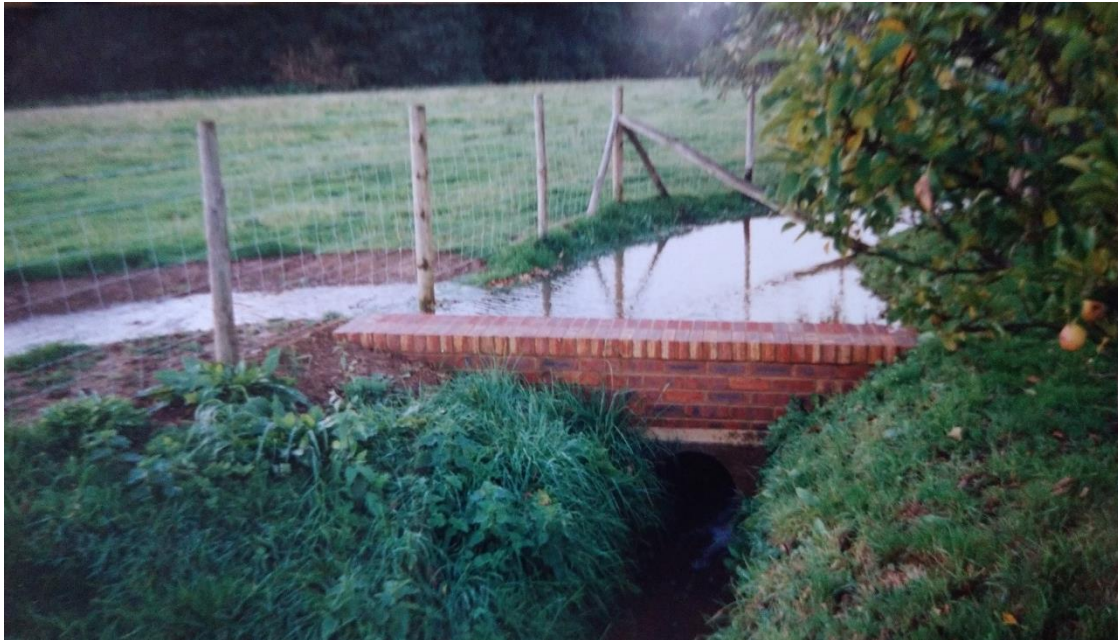
Figure 39. The resident of the most southerly house in the Alders Road cottages has erected a brick control structure many decades ago that diverts the flow of the ditch in times of peak flood to stop the ditch from being overwhelmed closer to the houses.
