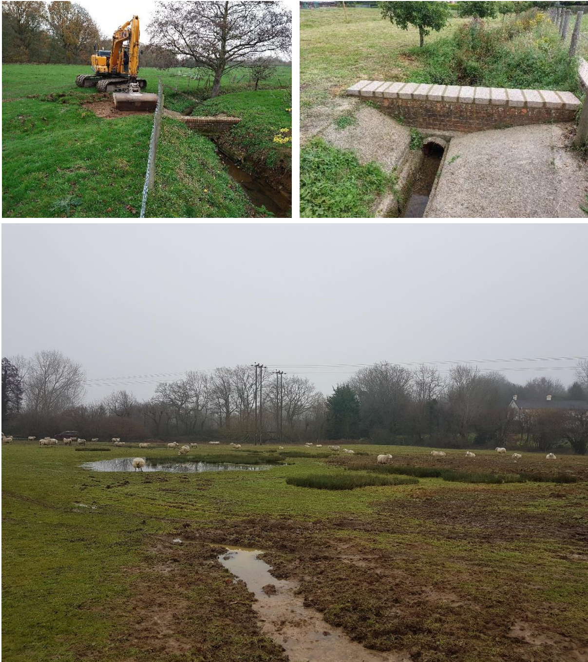
Figure 54. Top left: an excavator excavated an off-take channel from the brick control structure on the south side of the Alders Road cottages. Top right: extra layer of concrete blocks added to brick control structure. Bottom: the off-take flows into a scrape that was also dug out in a field used for pasture.
