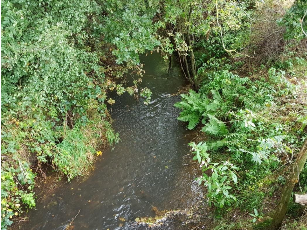
Figure 7. A deeply incised section of the Hammer Stream (a tributary of the Medway). The channel is disconnected from its floodplain for all but the most extreme flows.
