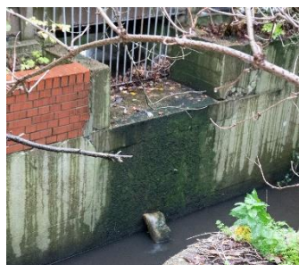
Epsom Storm Tanks
